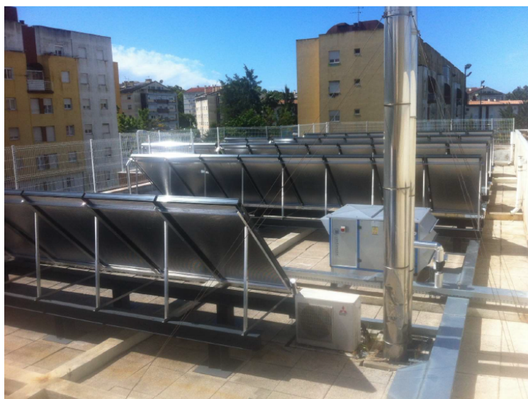
Figure 4. Solar thermal system installed in the pool roof. Source: Lisboa E-Nova.
